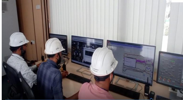
Plant control room (DCS, PLC, SCADA)
