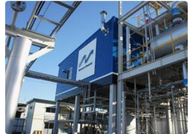
M3K, the world's first large-scale microwave chemical plant, completed in Suminoe, Osaka.
